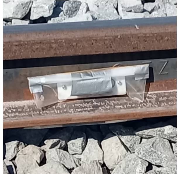
Figure 3.15 – Detailed View on the Position from Figure 3.14 with the Thermometer at the Rail Foot Partly Visible
