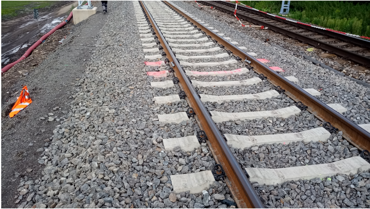
Figure 9 – Marking of Stationing with Measuring Spots in the Bezprávi Measuring Locality by Red Colour on the Upper Surface of Sleepers Outside the Track Channel and by a Flag Made from an Orange Reflective Vest.
