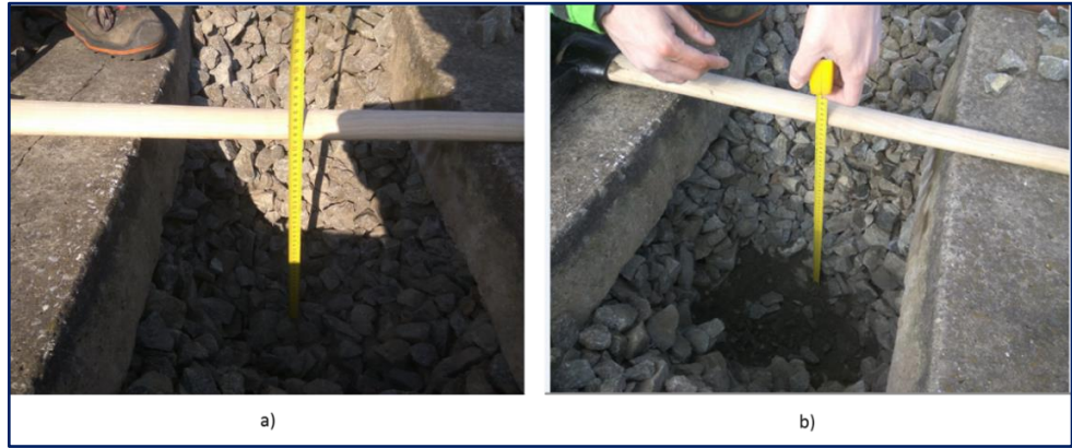
Figure 6.26. Trench 3: a) moderately clean ballast layer thicknesses measurement, b) moderately fouled ballast layer thicknesses measurement
