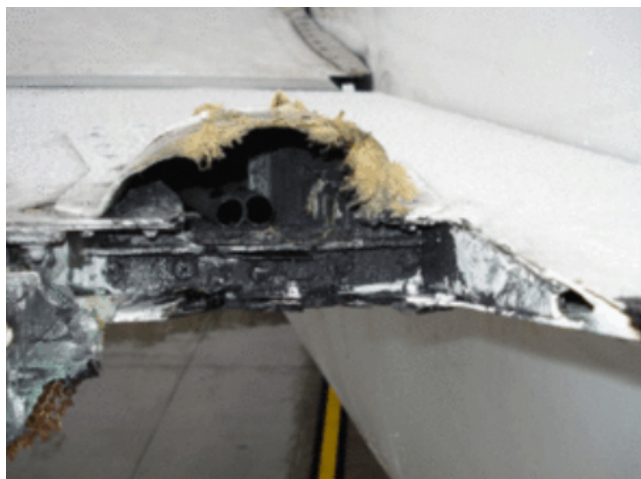
Figure 2. Damage caused by a bond failure [4]
