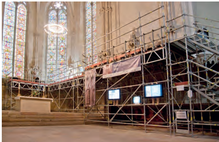
Fig. 7 Scaffolding installed for investigation in the west choir of Naumburg Cathedral. (Photo Dominik Jelschewski)
