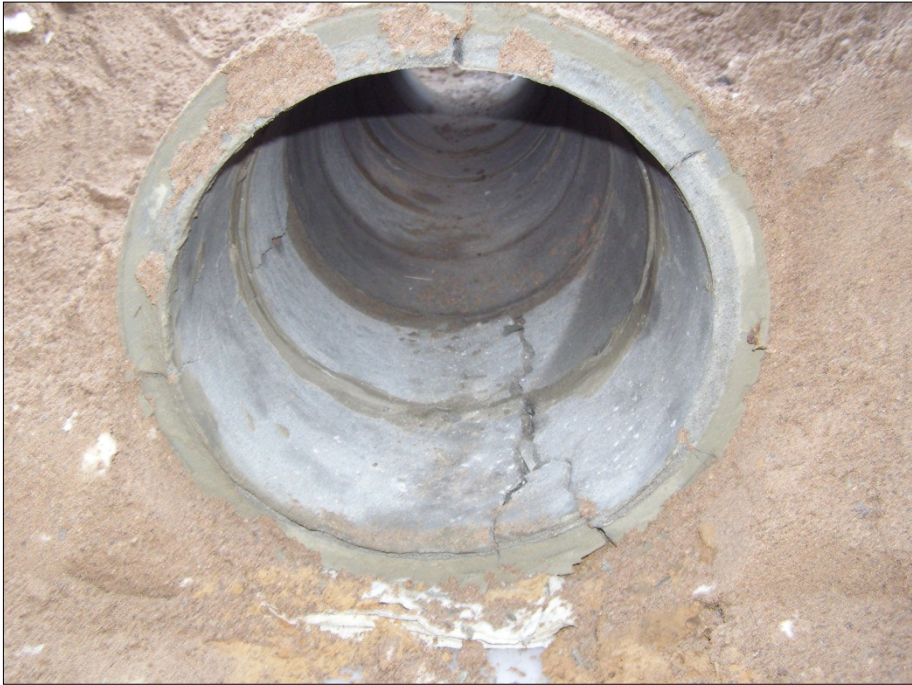
Fig. 8 Plain concrete after firing first bomb, the thickness of the cracks was maximum 11 mm
