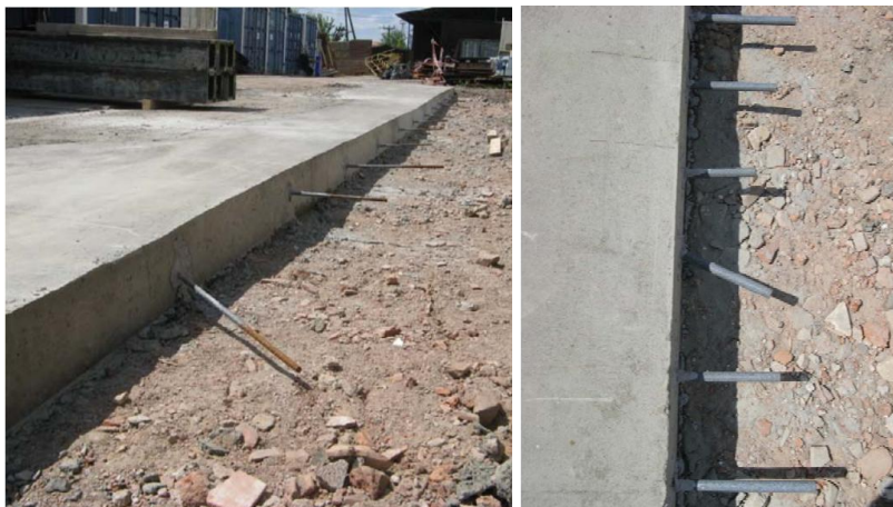
Fig. 5 View of the testing segment with in-built tie bars and top view on dowels
